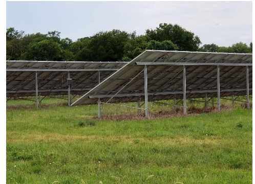
Example of a Solar Conversion System, Ground-mounted
