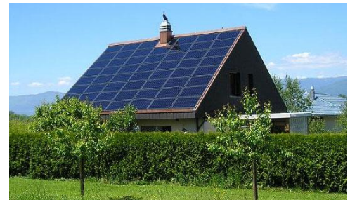
Example of a Solar Conversion System, Structure-mounted
