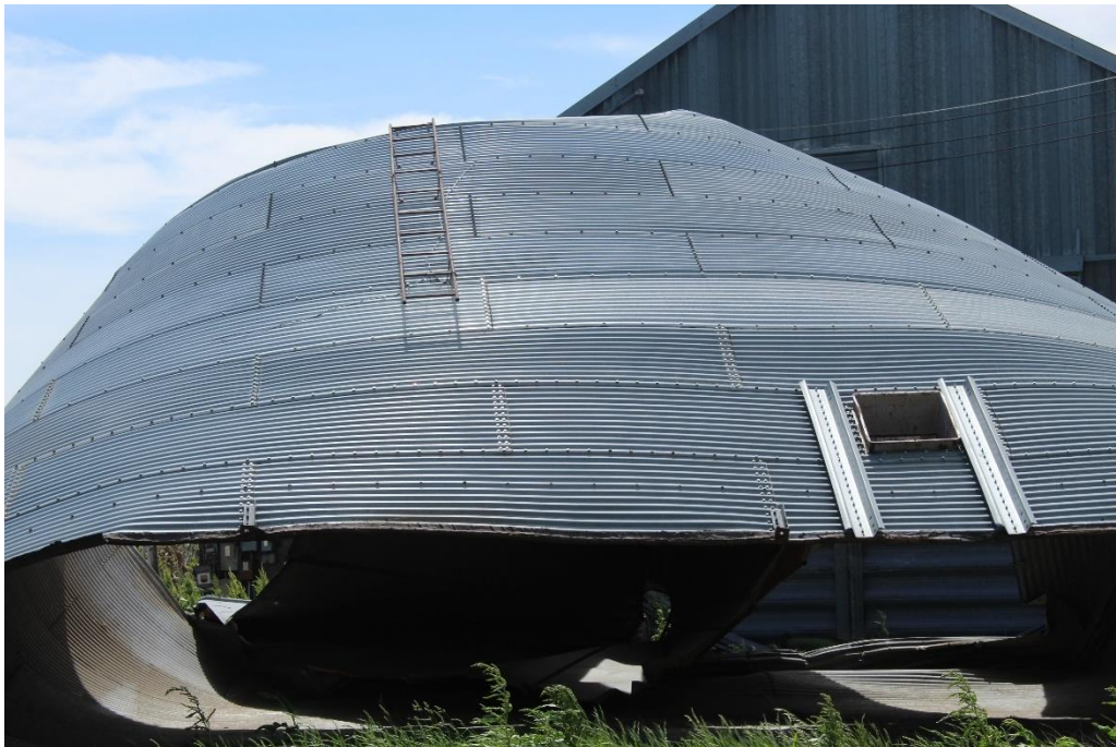
Deterioration of Sife or Other Improvements
